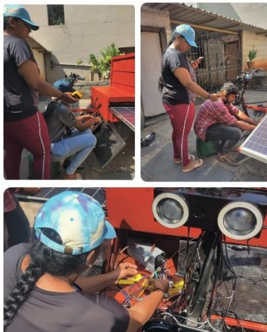
ELECTRICAL CONNECTION OF VEHICLE AND SOLAR PANEL
